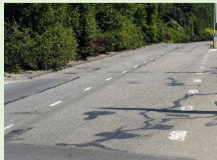
Scheurvorming asfalt (C)
