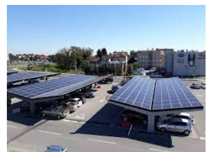
Figure 7 – Carport of solar panels
